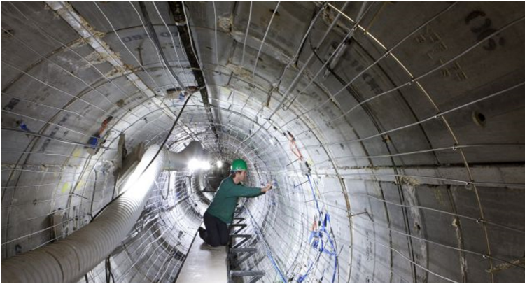
Fig. 8. Installation of the heating system for the PRACLAY Heater Test in the HADES URL. Source: courtesy of ESV Euridice.
