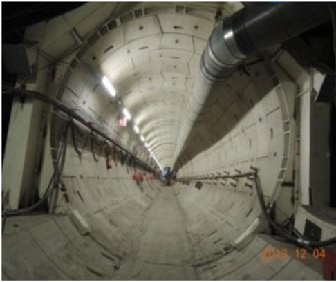
Fig. 8. View of the GRD4 gallery with the segmental concrete lining (Armand et al. 2015).
